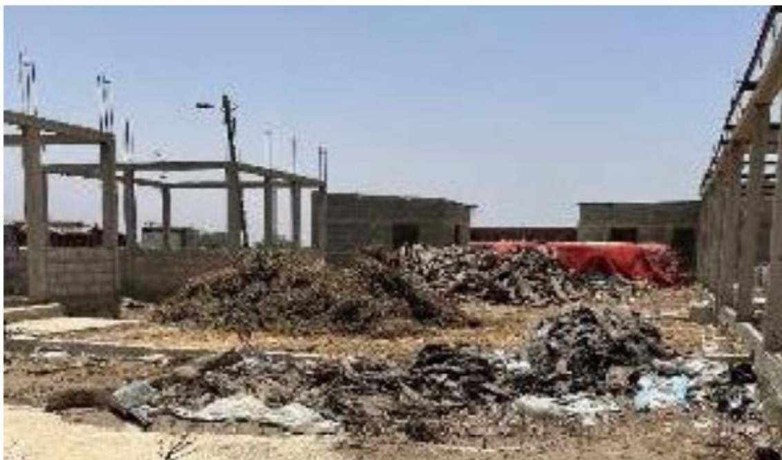
Photo 5. Reminders of construction site of the modern fish drying platform. Source: The Energy Consulting Group, July 2022.
